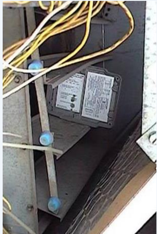
Notice the device that is supposed to be opening and closing the dampers has been jammed into the dampers, negating savings and creating huge energy waste in both the summer and the winter!
